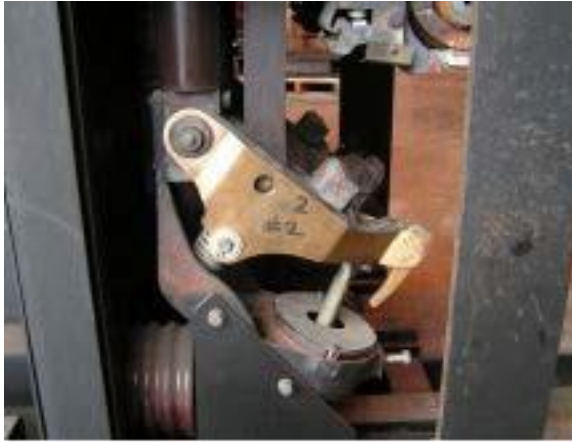
Figure 29. Installed Contact Assembly
