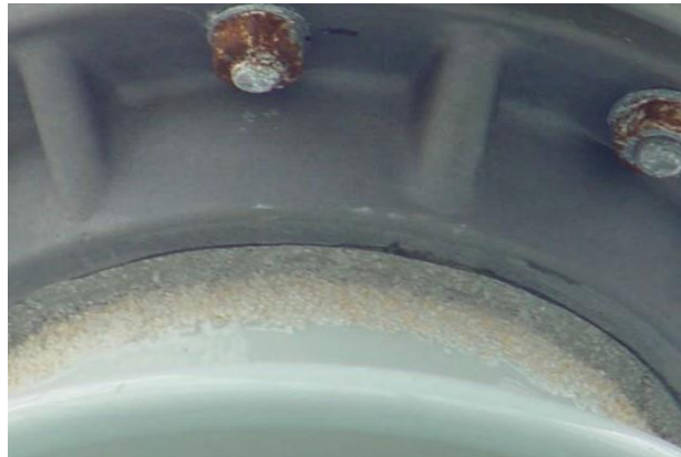
Figure 57. Possible Corrosion on Top Bushing Cap Hardware for Certain MEPPi SF 6 Breakers
