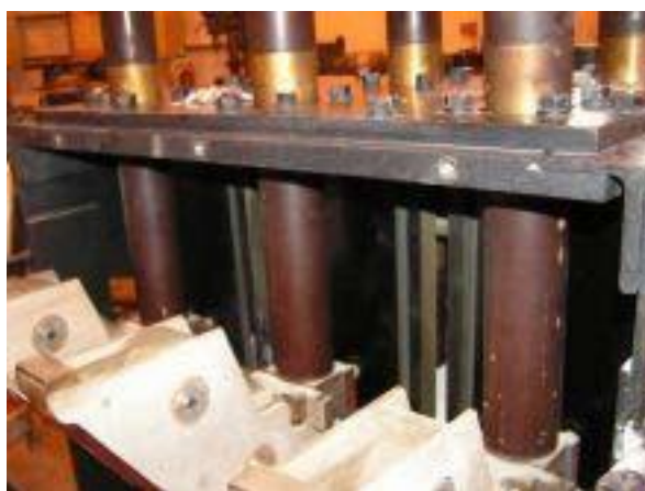
Figure 23. Load-Side Stabs and Separators
